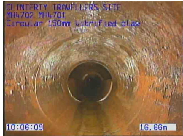
MH4702X_746f3fc1-433b-49d8-96be-4cddc50edb31_20230220_213221_512.jpg, 00:06:19, 16.66 m Fracture, circumferential from 12 o'clock to 12 o'clock
