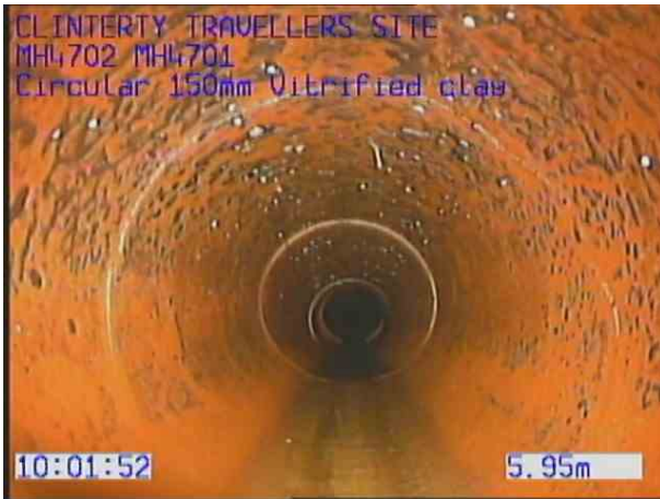
MH4702X_327954b5-d448-4682-b75a-2287ab7150c3_20230220_213106_968.jpg, 00:02:22, 5.95 m Crack, circumferential from 8 o'clock to 4 o'clock
